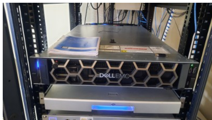
New Server Mounted in Rack
